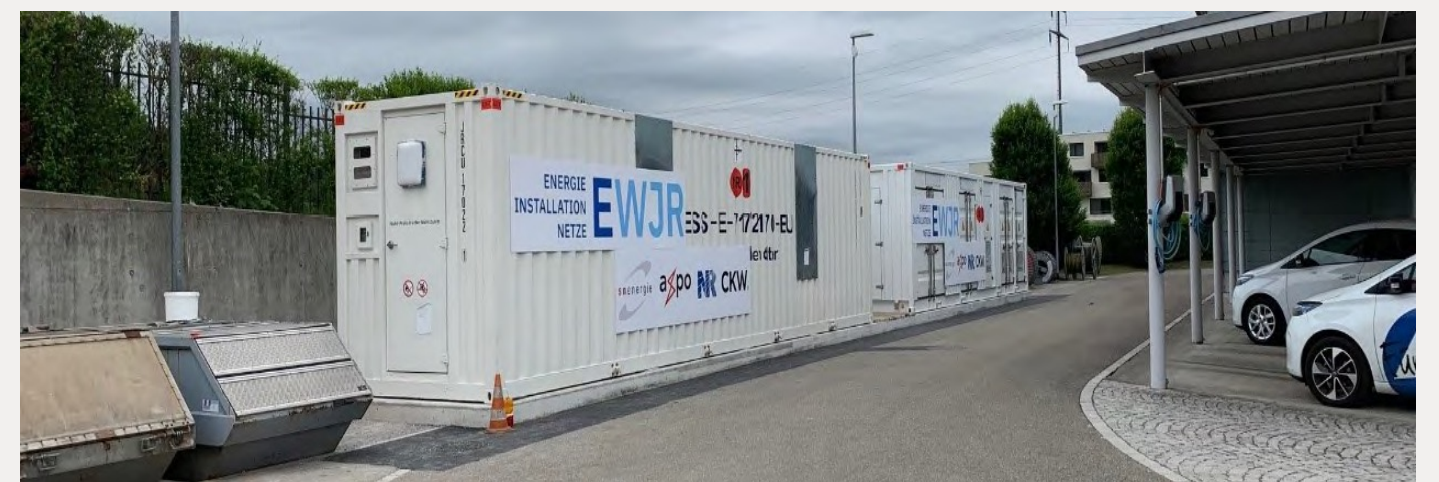
2MW/2.17MWh EWJR lithium battery energy storage project, Switzerland
