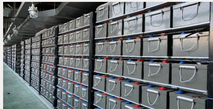
12MW/48MWh Jinling Station Lead-acid Battery Energy Storage Project Huzhou, Zhejiang
