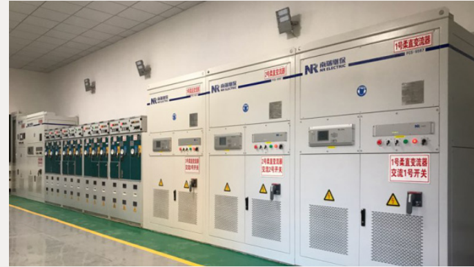
300kW/340kWh Low-voltage flexible distribution network lithium battery energy storage + DC distribution network converter project Xuzhou, Jiangsu
