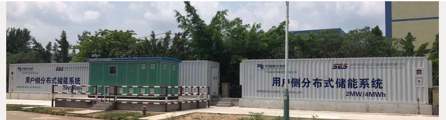
2MW/4MWh User side lithium battery energy storage project, Conghua, Guangdong
