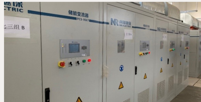
12MW/48MWh Baililian Lithium Battery Energy Storage Project Jiaozuo, Henan
