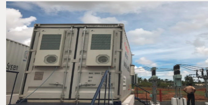
1MW/0.5MWh India Power Grid first energy storage system, India
